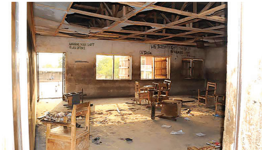
Dilapidated Public School, Nigeria
